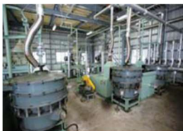
Waste oil treatment (vibration sieving machine)
