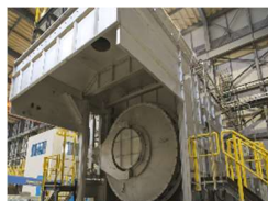
Waste lead melting process (rotary gas melting furnace)
