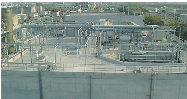
Activated sludge processing facility for biological treatment of wastewater (Daiseki Nagoya Works)
