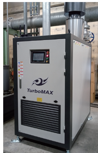
Turbo blower in the activated sludge facility (Daiseki Kanto Works)
