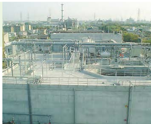
Daiseki Nagoya Works' activated sludge treatment facility
