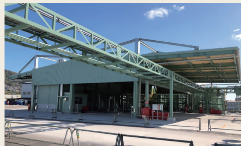
Supplemental fuel plant at Kyushu Works
