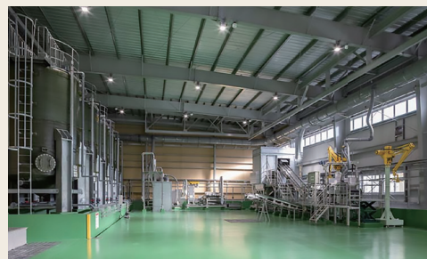
Industrial waste treatment facility at Daiseiki MCR's Hiraide Plant
